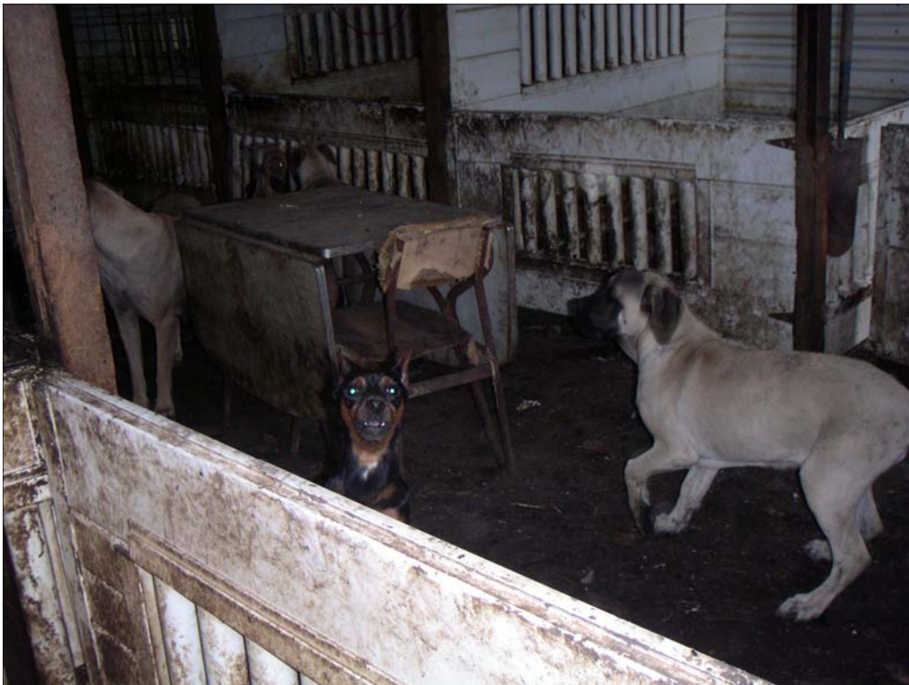
Filthy Pens in Whelping Building; Discarded Chair and Table
