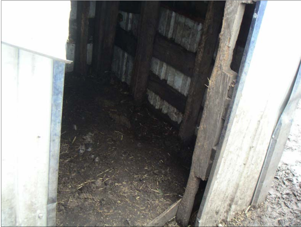
Dirty Whelping Building with Worn Wood
