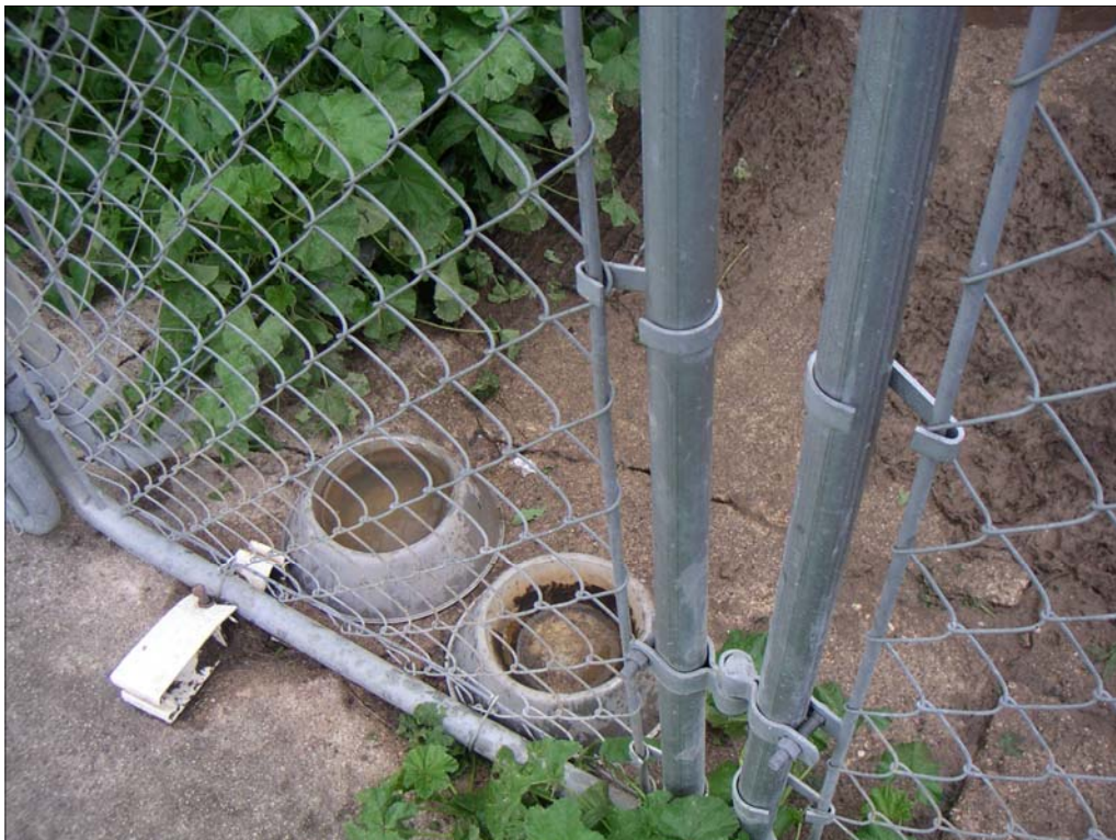
Cracked Concrete and Weeds; Rusty, Dirty and Empty Food and Water Bowls; Mud and Feces
