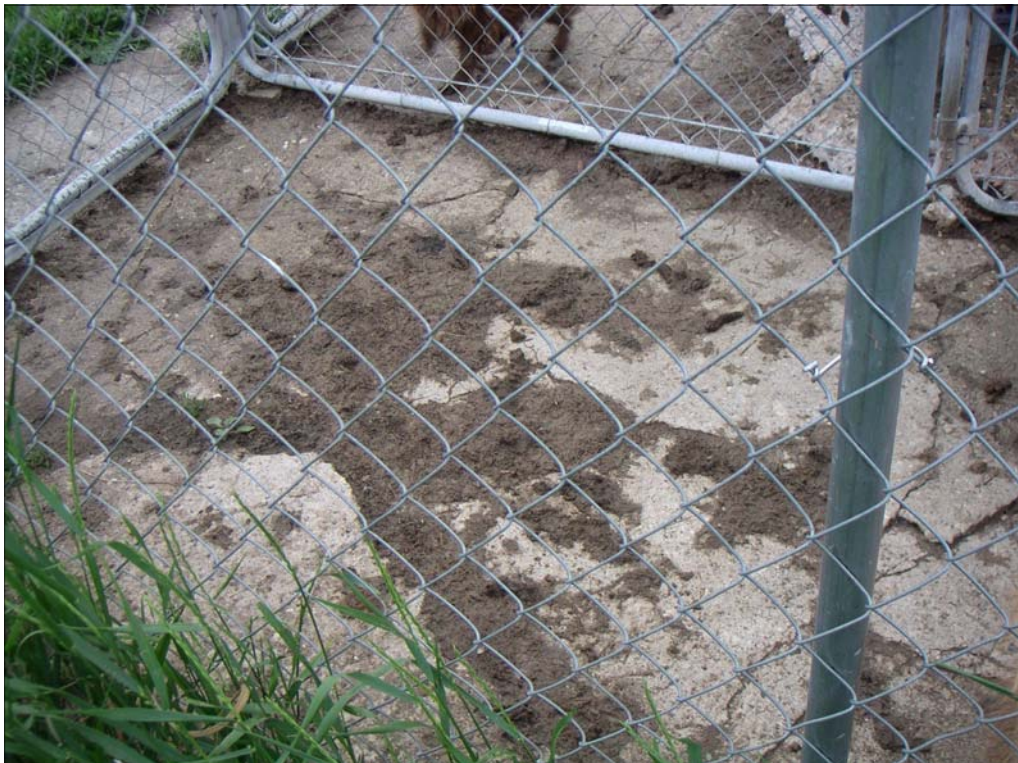
Mud, Feces, and Weeds; Cracked Concrete
