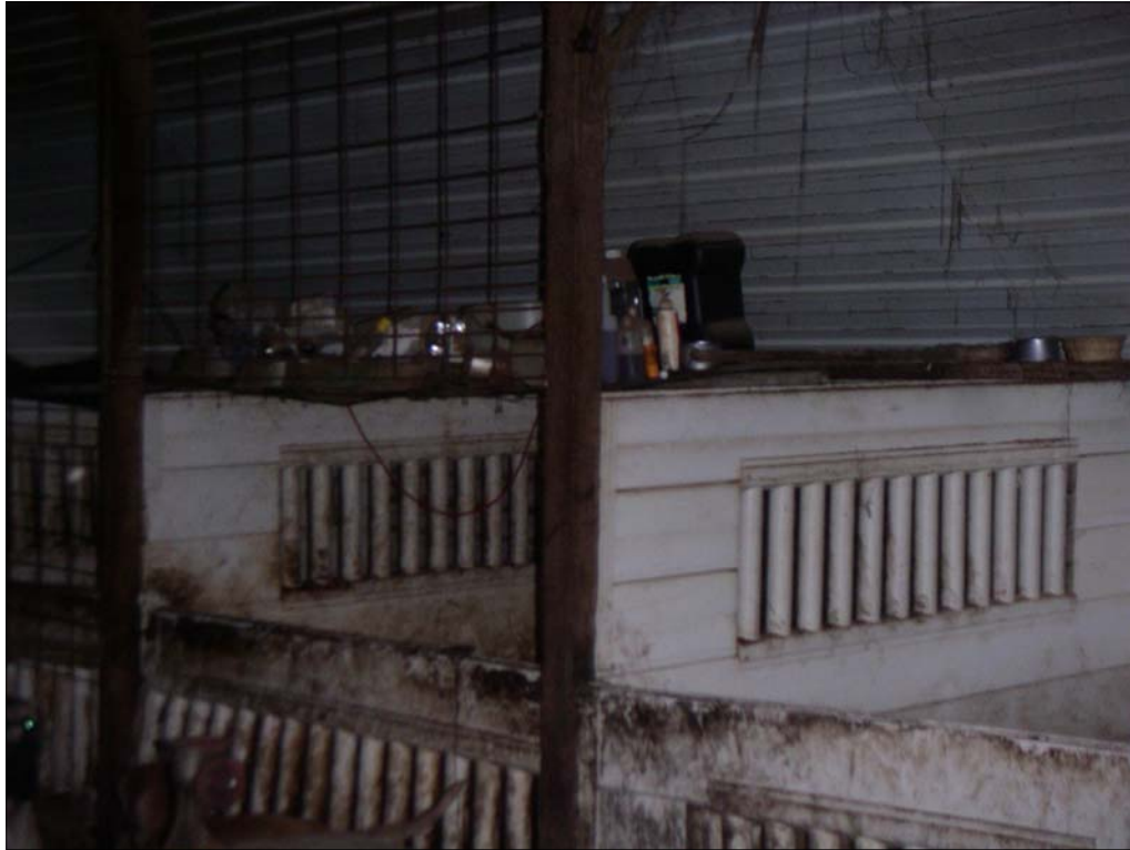
Filthy Pens in Whelping Building; Clutter
